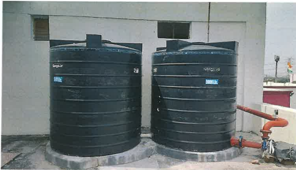
Site photograph 2 Water Storage Tank in Campus
