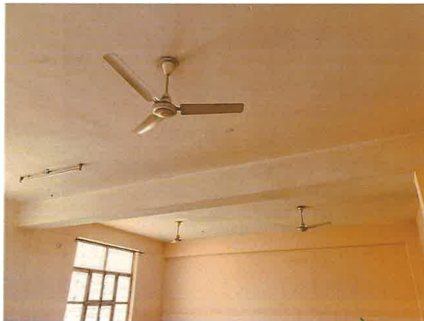
Site photograph 1 Classroom conventional fan
