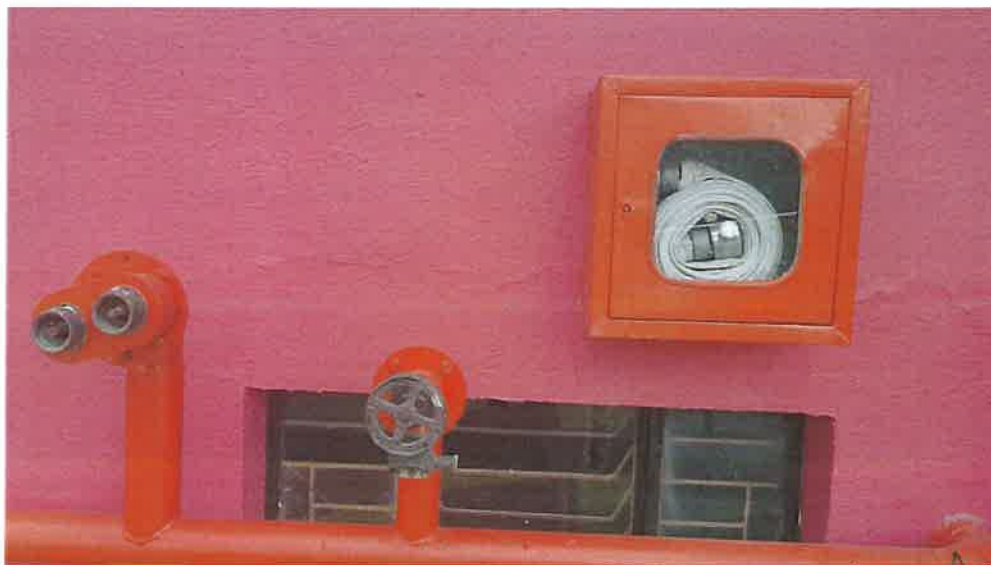
Site photograph 4 Fire Safety Pipeline and Hose
