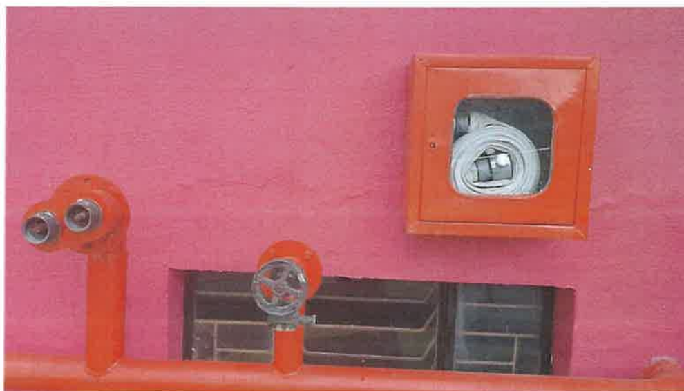
Site photograph 4 Fire Safety Pipeline and Hose
