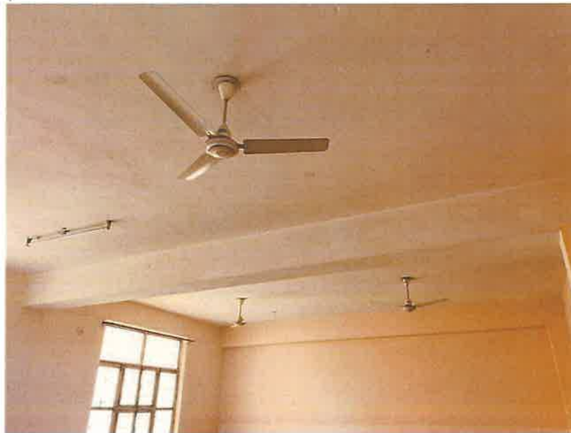
Site photograph 1 Classroom conventional fan
