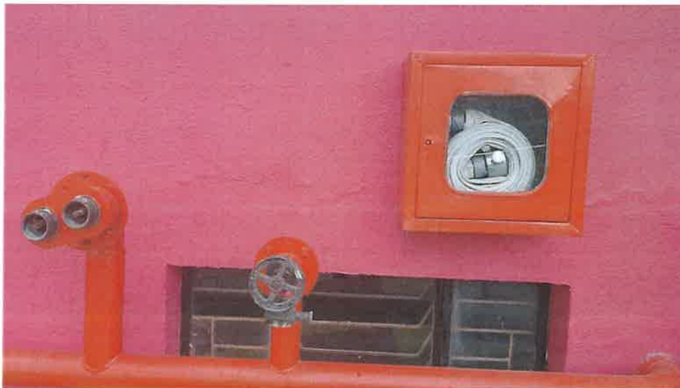
Site photograph 4 Fire Safety Pipeline and Hose
