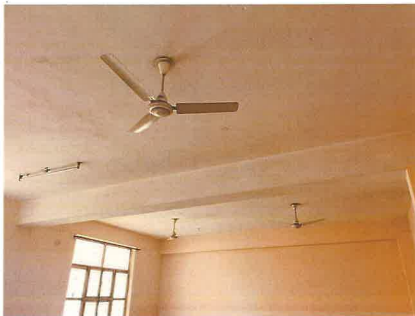
Site photograph 1 Classroom conventional fan
