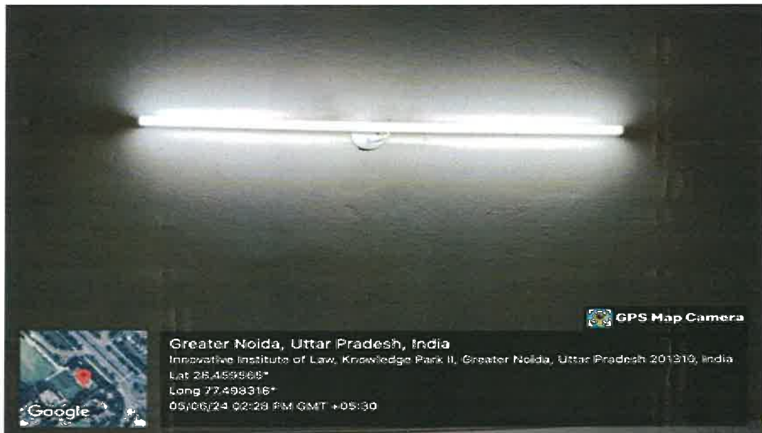
Power-Efficient LED Light in IQAC office
