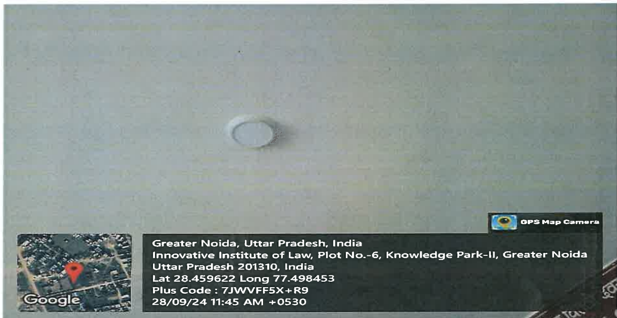
Power-Efficient LED Light in Corridor
