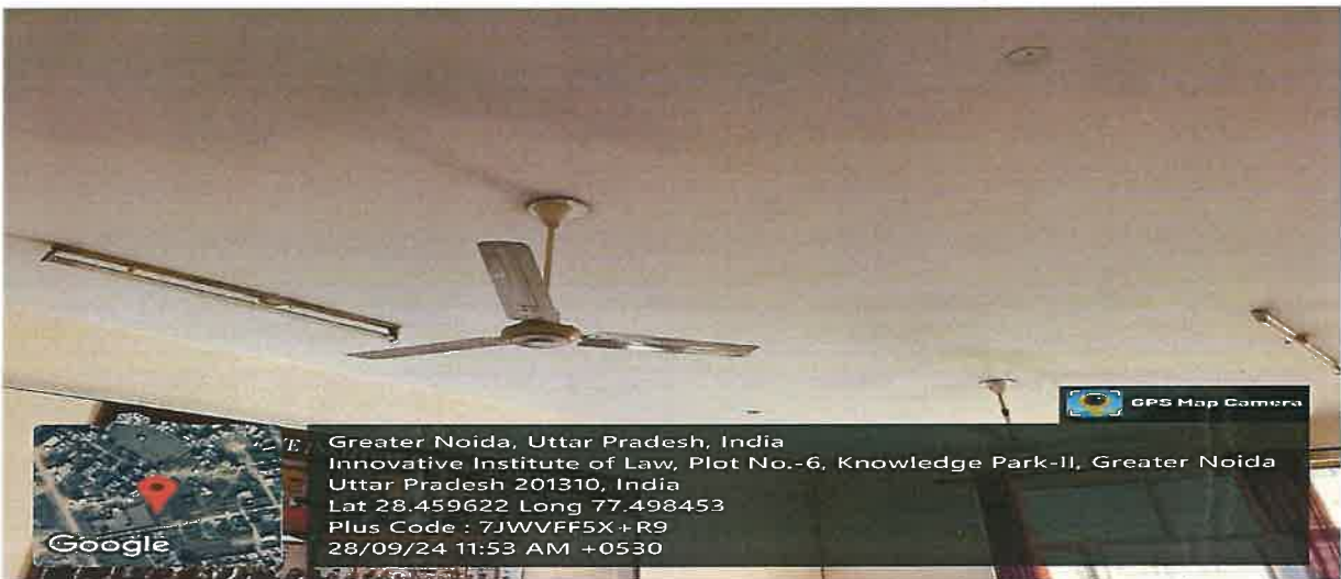
Power-Efficient LED Light in H.O.D Office
